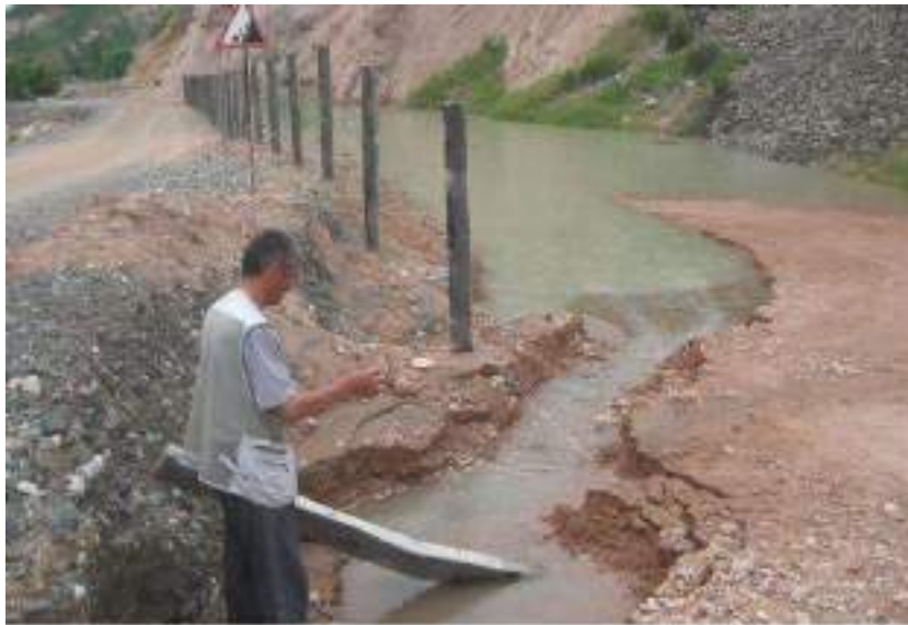
Radioactive landslides broken fence
